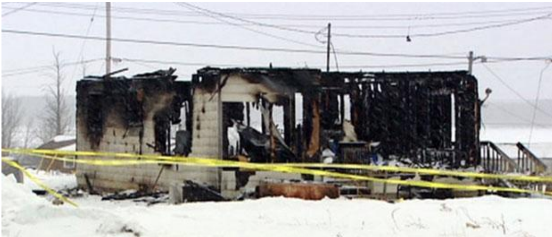
A house on God's Lake Narrows First Nation was reduced to rubble after a fire (CBC)
